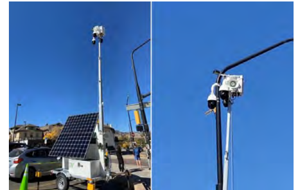
Parking Lot with Security Camera in Boulder, CO
