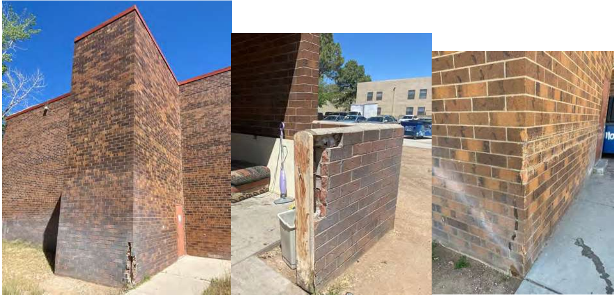
Structural Wall Deficiencies (Wainwright Manor)
