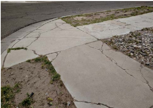
Crumbling sidewalk from shifting land underneath
