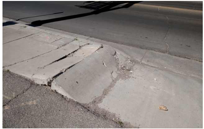
Buckling sidewalk and pavement
