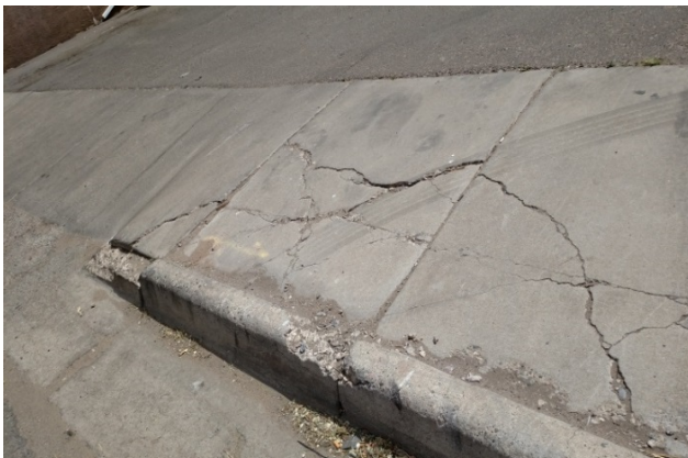
Crumbling sidewalk from heavy vehicles
