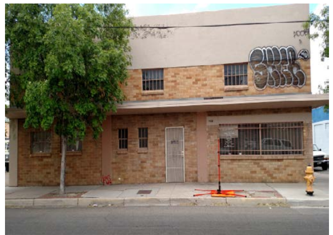
Building façade needs to be cleaned
