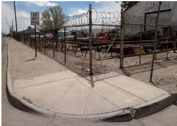
Accessible ramp with no connecting sidewalk
