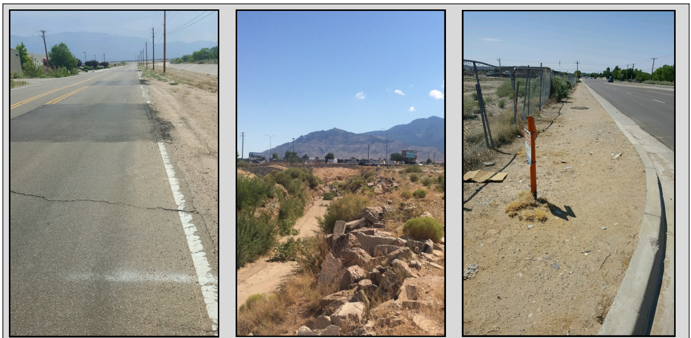
Figure 3. Infrastructure Deficiencies in the MR Area. From Left to Right: Expanding and Contracting Road Conditions, Deteriorating Drainage Channel, Lack of Sidewalks
